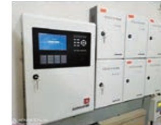
Flammable gas warning system
