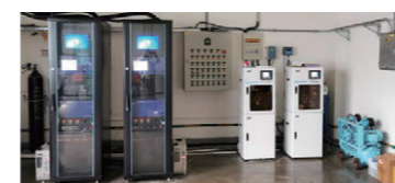
Online emissions monitoring unit
