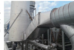
Water circulation line for the painting booth
