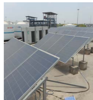
Solar panels that have been installed
