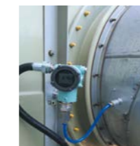
VOC measuring facility
