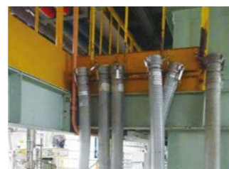
Connected hoses separately identified
