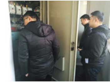
The electricity monitoring system that was installed
