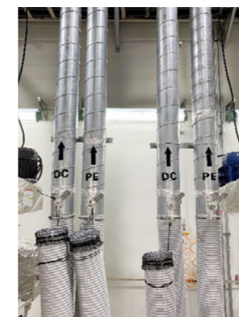
Separated exhaust ducts
