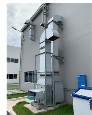
Exhaust treatment unit
